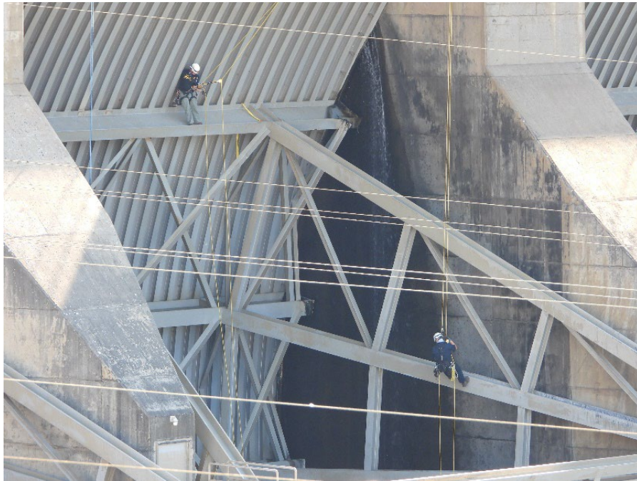
Figure 1: An inspection of the tainter gate at spillbay #3 (Note: the horizontal lines are not associated with the inspection; they are avian lines).
